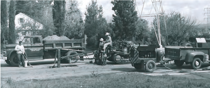
Many of the pipes installed in the 1950s and 1960s (like those shown above) may need to be replaced.
