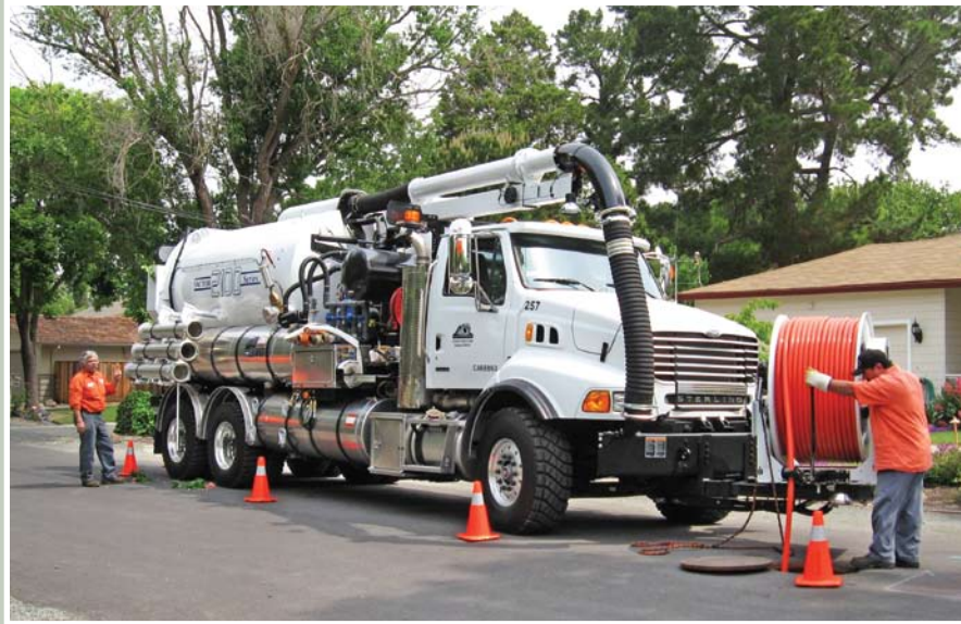
This large truck is known as a Hydro-Vac. It uses a high-pressure water spray and a variety of nozzles to clean grease and other built-up materials from the inside of sewer pipes—and a vacuum to remove the debris.
