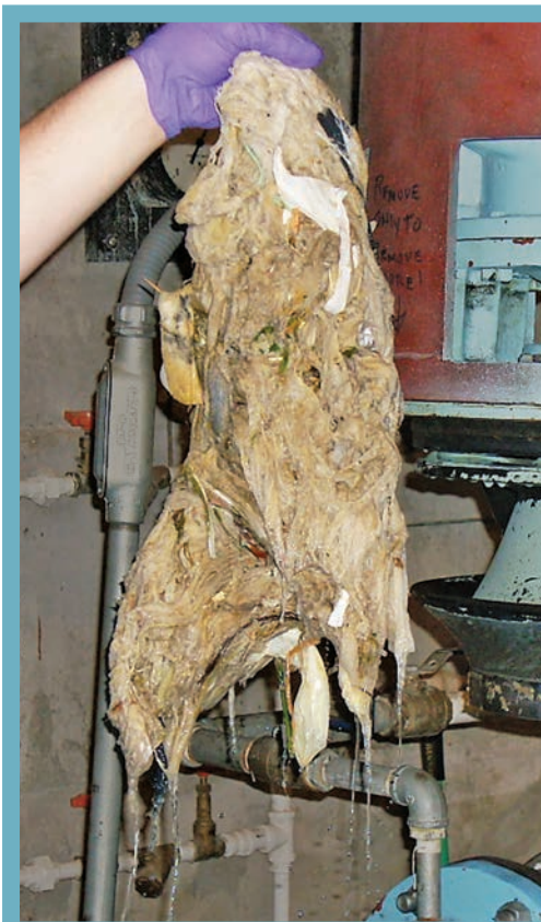
A clump of wipes like this can clog sewer pipes in your neighborhood!
