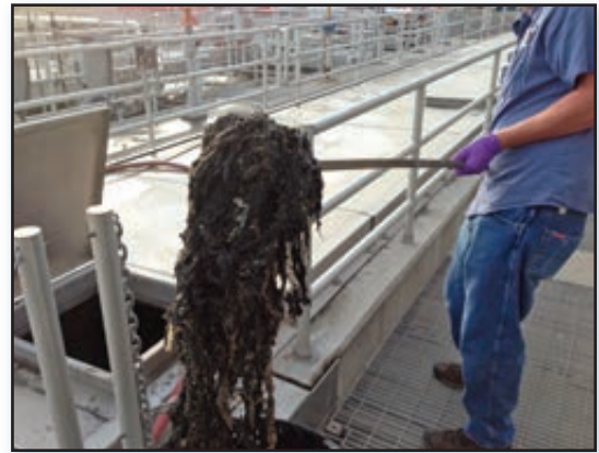
Wipes flushed down sewers clog equipment at our treatment plant.
