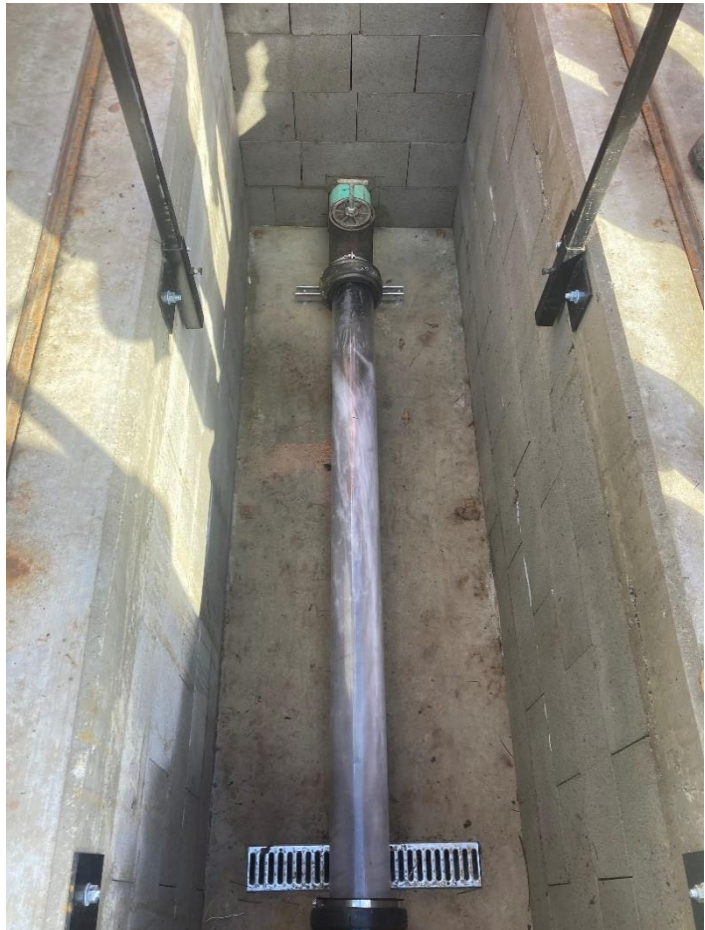
Figure 4.10: – Pipe O&M Training Vault at CSO Facility
